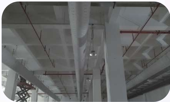
Chongqing Huasen Pharmaceutical (Rongchang) Pharmaceutical Cooling warehouse
