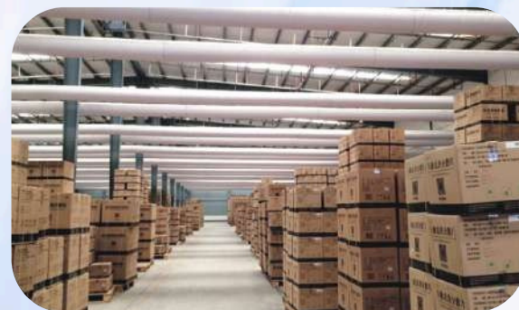
China Merchants (Zhengzhou) Pharmaceutical Cooling Library
