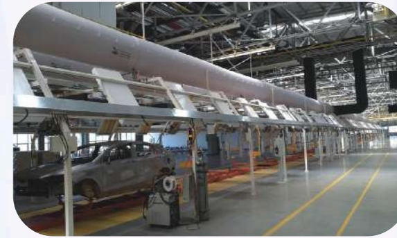
Beijing Automobile (Zhuzhou) Phase II Huizhuang Workshop
